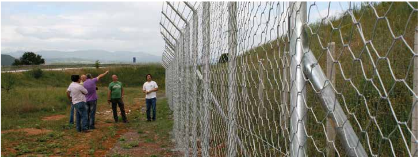
Fig. 9. Installing the “bear-proof” reinforced fence on the highway after successful efforts of CALLISTO.
